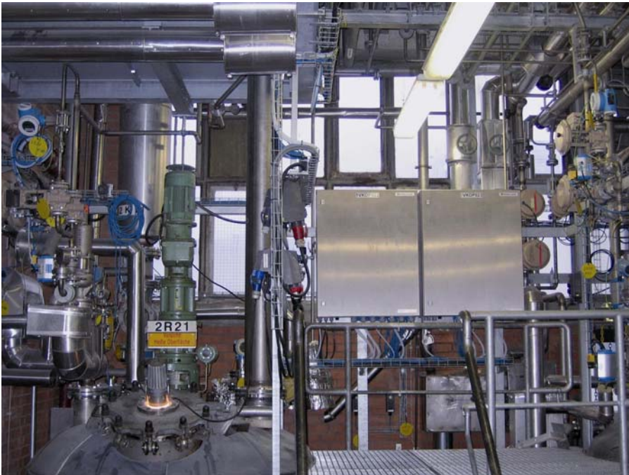
Fig. 1: Part of the plant with associated RPI switch cabinet
